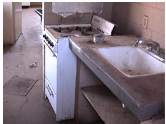
At least 25% of the government sponsored farm worker housing in the Panhandle such as this apartment in Floydada, Texas is in poor condition.
