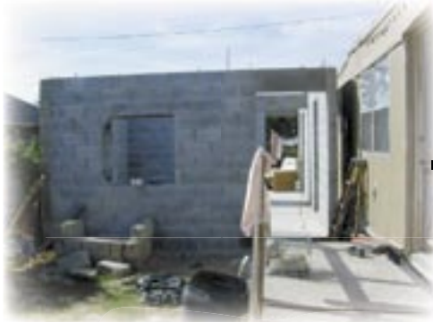
2003 photo - Family lives in the mobile home as they build three rooms of concrete blocks next door.
